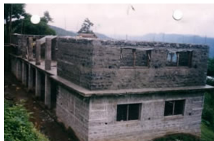
HeNN provided fund for the reconstruction of this school in Sudal Village, Bhaktapur
