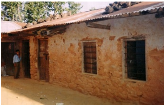
Kanyadevi School in dilapidated condition
