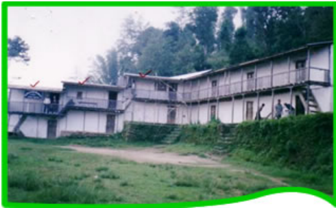
Sankhuasabha school in disrepair
