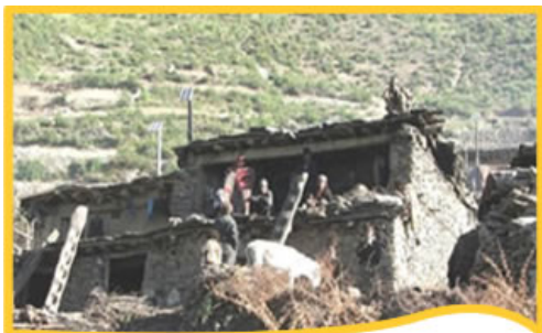
Solar panels on the rooftop in houses in Humla
